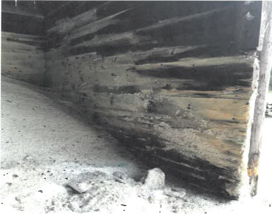
Photo 5: Belmont (314)- Deteriorated wall condition
