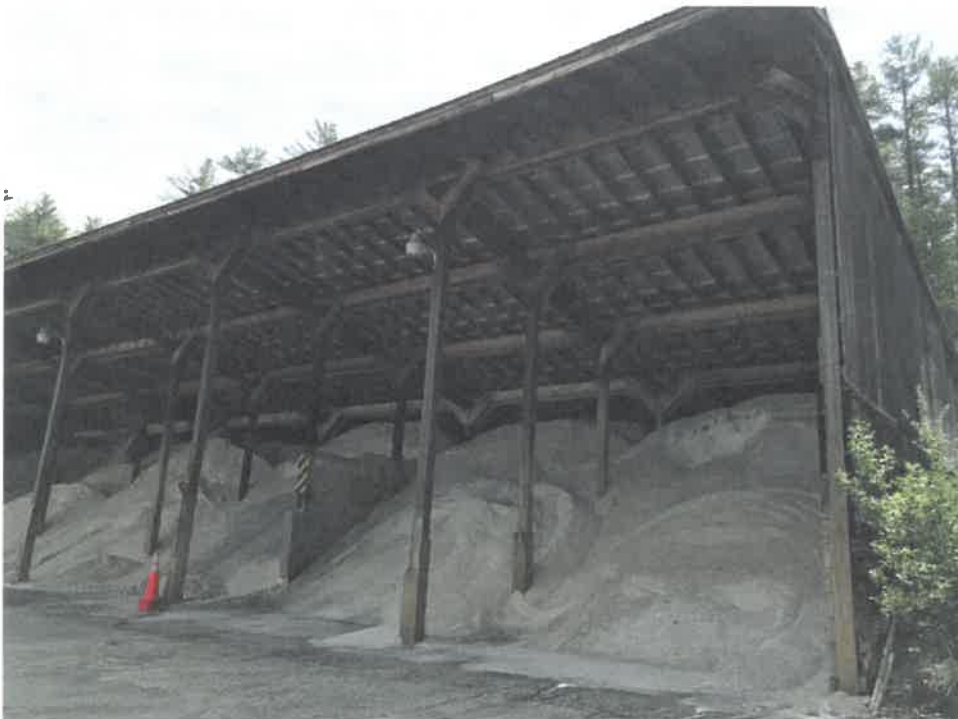
Photo 6: Warner (526) – Salt Shed inadequate capacity
